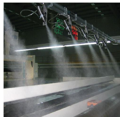
喷雾加湿 Spraying humidification
