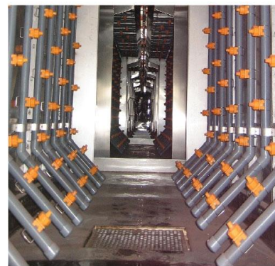
喷淋室 Spraying room
